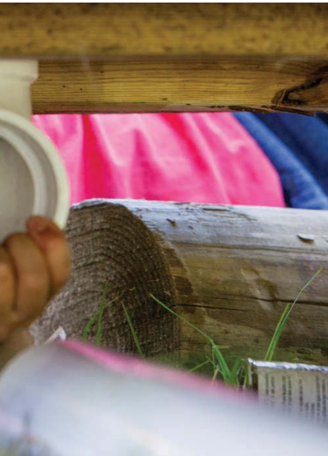
▼ Josh Jackson installs a new 4-inch PVC drainline below the floor of a cabin.
