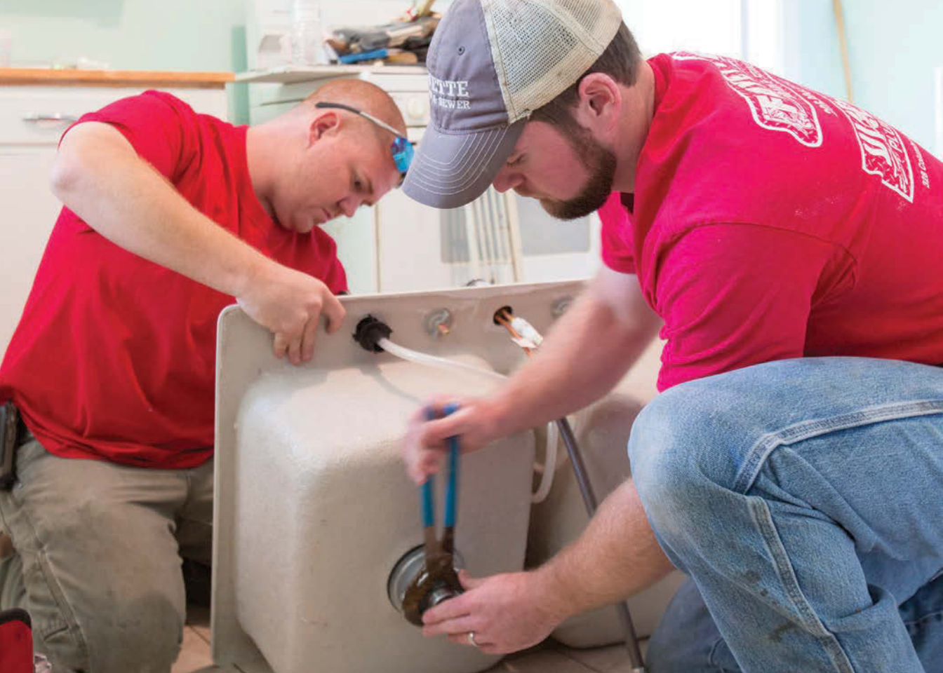
Shawn Leonard (left) and Justin Simmons install the plumbing on a new sink before setting it in place.
