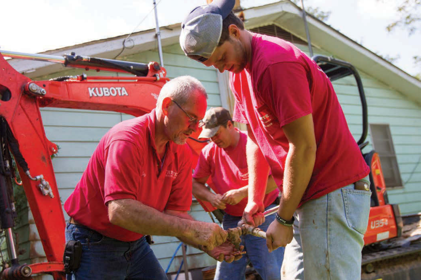
Jeff Goree, Josh Jackson and Harrison Kummer (from left) work on a waterline repair outside a home in Fayette, Alabama.
