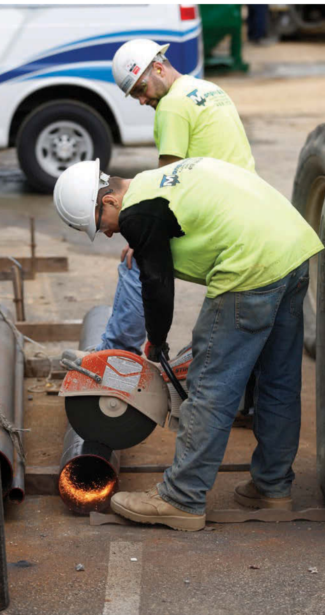
▲ Matt Cornwell (front) and Luke Day use a Stihl cut-off saw to cut pipe for a rain conductor system on a new commercial building.
