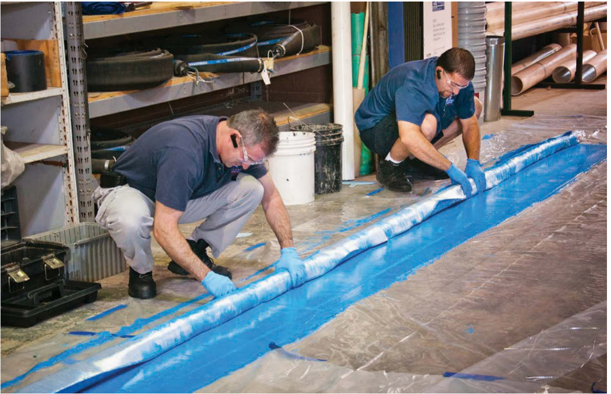
▲ When strong sewer odors threatened to close a newly remodeled office building and displace its occupants, Levine & Sons inspected the pipes and was able to solve the problem with a Formadrain sewer liner.
