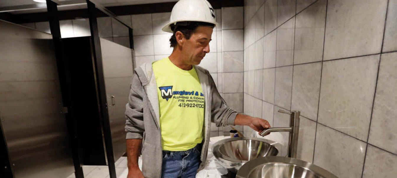
▲ Plumber Mark Kramer tests the rotation on one of several new fixtures in a public bathroom.
