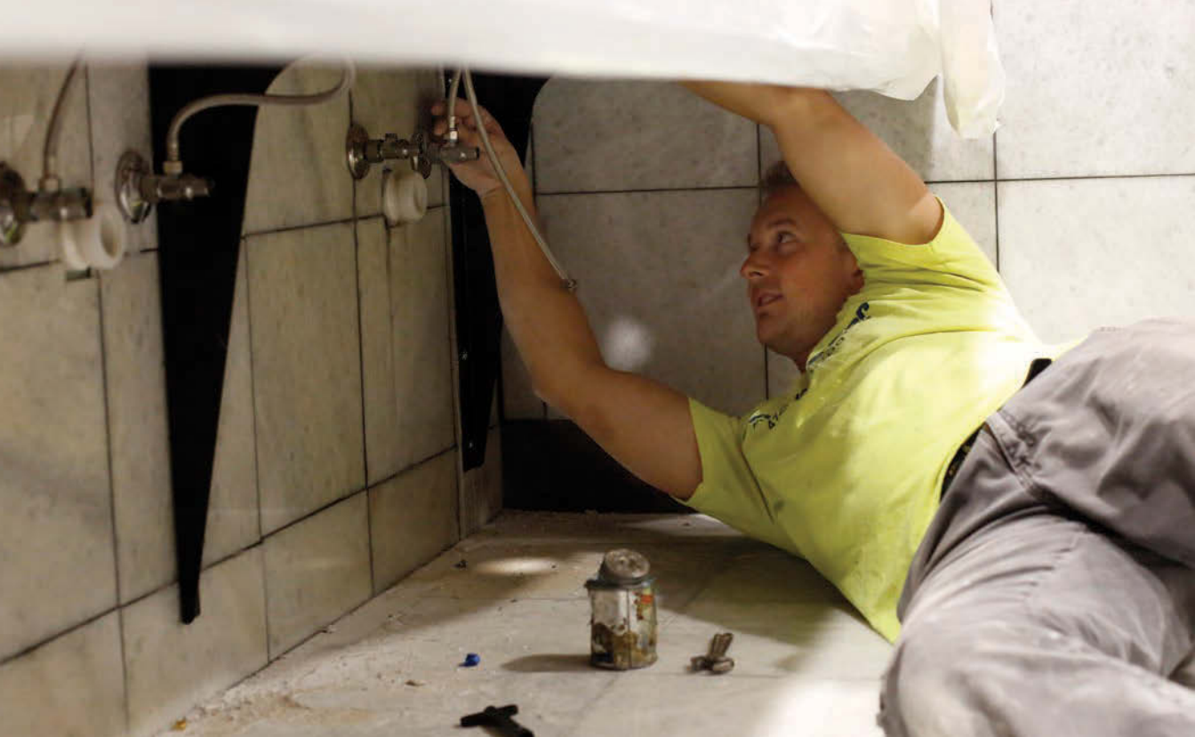
▲ David Lemak hooks up the supply lines on a row of new sinks in a Pittsburgh commercial building's public bathroom.
