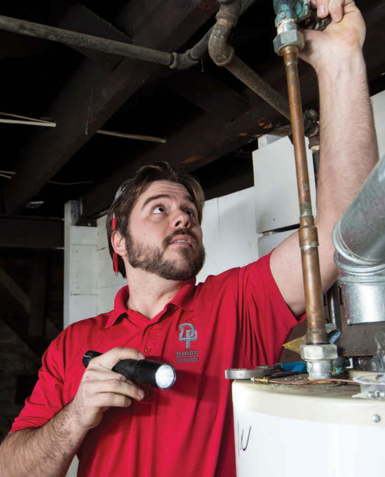
◀ Plumber Matt Koenig shuts off a water supply line (top) before removing a garbage disposal (bottom) to make room as he prepares to install a shut-off valve for a new dishwasher.
