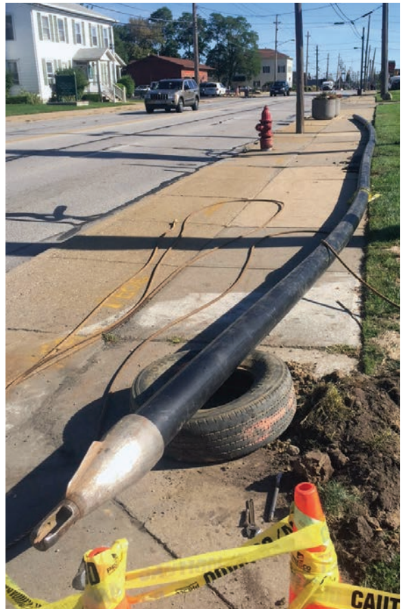
▼ Campbell's quick and effective response led to more work at the dealership, replacing the old 4-inch cast iron sewer line with 160 feet of new 6-inch HDPE pipe without tearing up the new parking lot.
