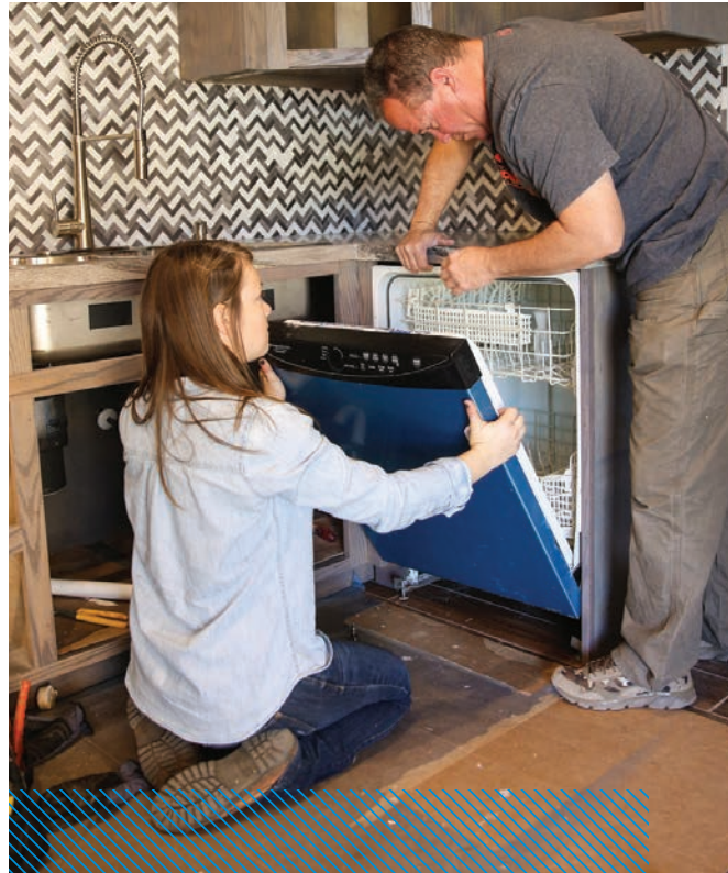
▲ Makenzie Johnson and contractor David White check the door closure and adjust the position while installing a new dishwasher.
