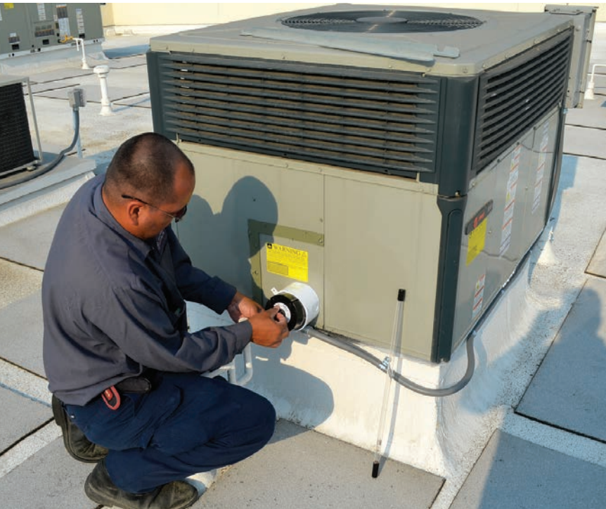
◀ A technician installs an X-Plus UV-C lamp in an air-handling unit. Applied in new systems, UV-C lamps prevent the buildup of organic material.
