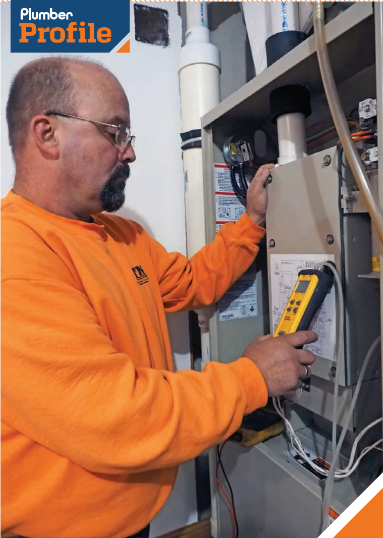
▲ HVAC-R technician Mike Maas restores heat to a home after checking the furnace gas pressure and wiring components.
