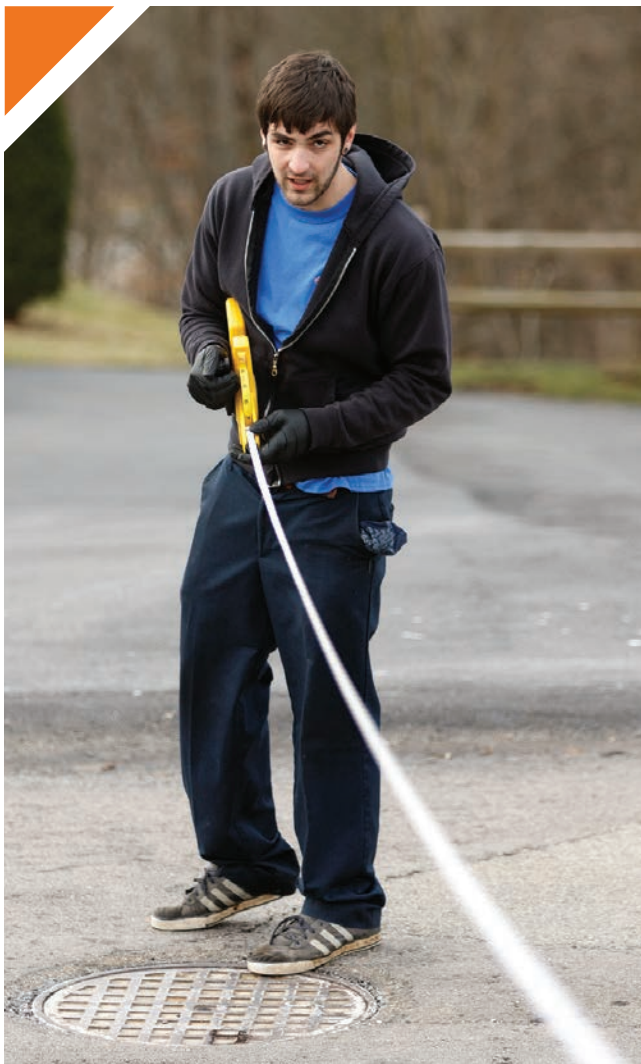
▼ Caleb Graft measures the distance from where the home’s sewer connects to the mainline.
