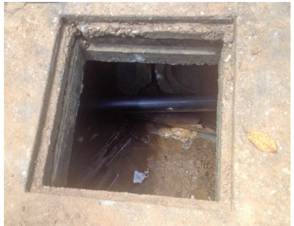
▲ The 4-inch HDPE pipe advances through the enlarged holes in the concrete stormwater vault. Behind the pipe are two 36-inch-diameter concrete drains. The original clay tile lateral switched to cast iron at this point.
