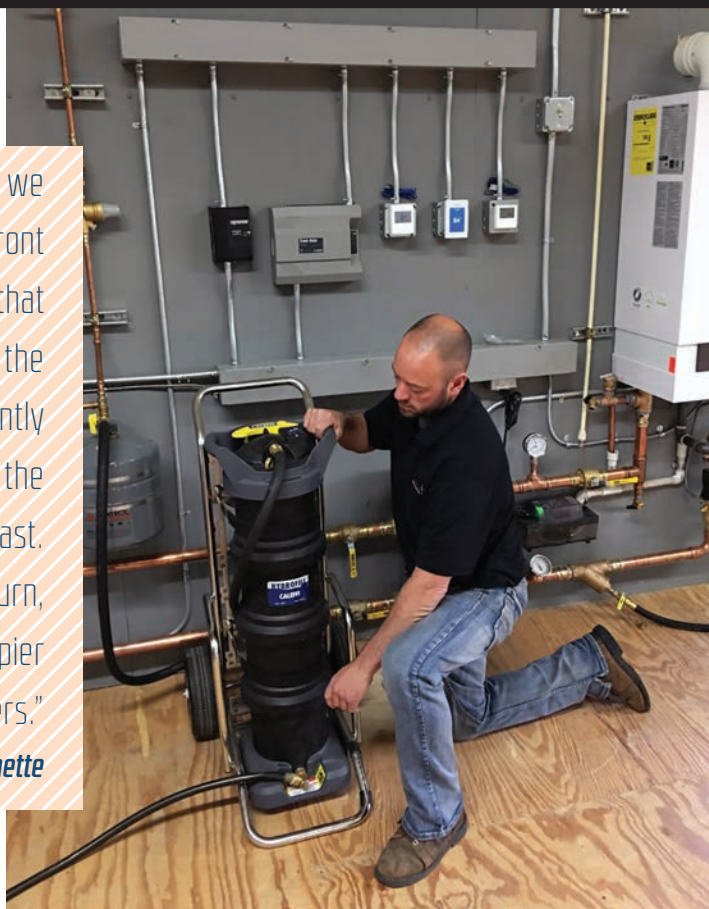
▲ Tim Pederson, lead hydronic expert for Cardinal Heating & Air Conditioning installs a Hydrofill NA570924 water-treatment unit at a commercial job site near Madison, Wisconsin. The unit removes minerals from water to make it better for the hydronic boiler systems.
