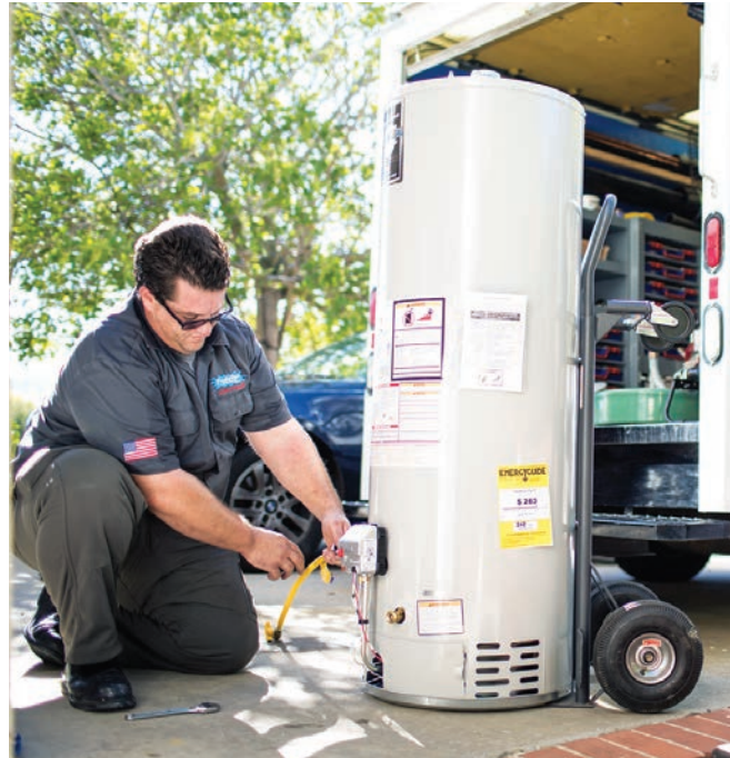
▲ Pacific Drain & Plumbing service technician Ryan Colgan preps a new water heater for installation in a client's driveway. The California-based company relies on word-of-mouth when it comes to marketing the business. (Photography by Collin Chappelle)
