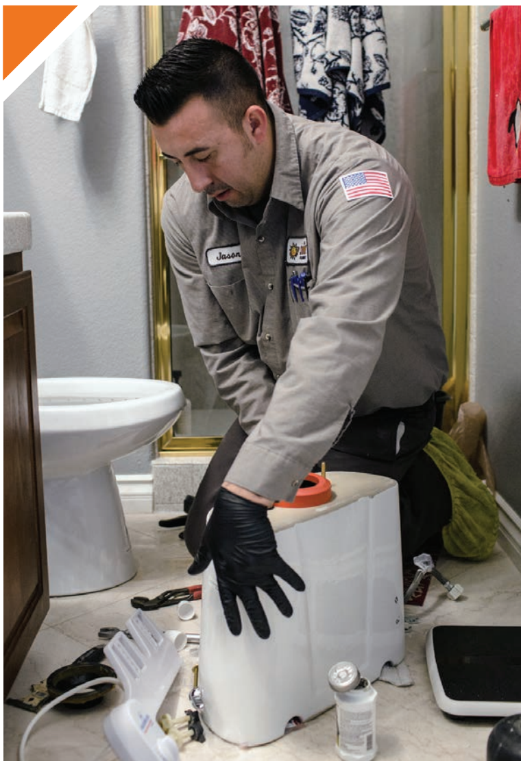
► Plumbing technician Jason San Roman works on a new toilet installation at a home in Las Vegas.
