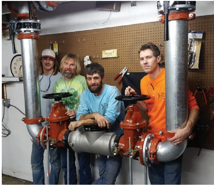
▲ The staff that worked on the backflow prevention valve were Taylor Votion, Josh Mason, David Wright and Mike Wells.
