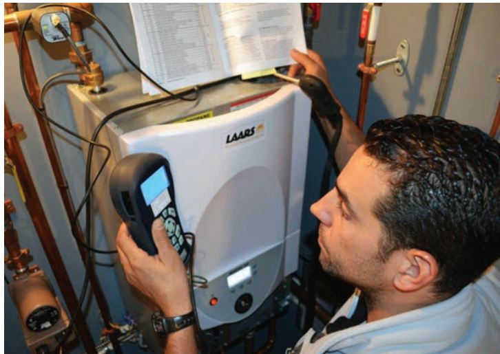
▲ Anthony Tosco, owner of Avanti Plumbing, Heating and Cooling in Audubon, Pennsylvania, uses a combustion tester to measure the combustion efficiency and carbon monoxide levels on a Laars Mascot mod-con boiler.
