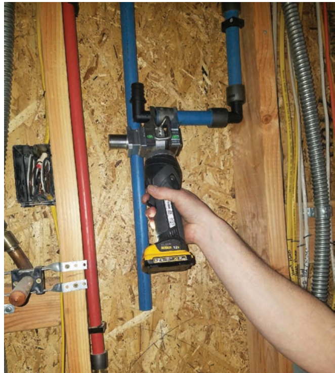
▲ Northwest Plumbing Services plumber Ron Blankenship uses a PEXa/EVERLOC+ compression-sleeve fitting system while on a new home installation job in Bellingham, Washington. (Photos courtesy of Northwest Plumbing Services)
