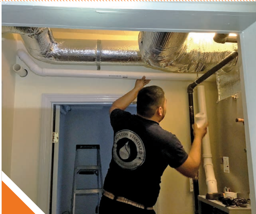
▲ A plumber from Boston Standard Plumbing and Heating assembles PVC pipe in a home where crews were met with tight crawl spaces. (Photo Courtesy of Boston Standard Plumbing and Heating)
