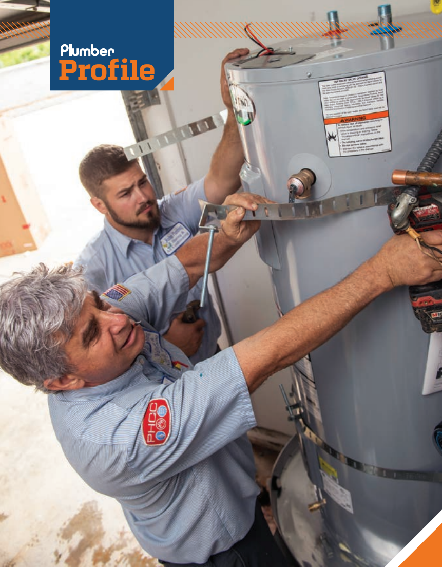
▲ Bob Hollowell (front), journeyman, and Caleb Castle, apprentice, secure the hot-water heater (A. O. Smith Water Heaters) in place with a drill (Milwaukee Tool).
