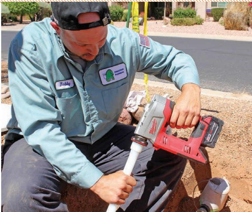
▲ Bobby Scirica uses a M18 ProPEX expansion tool (Milwaukee Tool) to expand the end of the new water pipe for the fitting.
