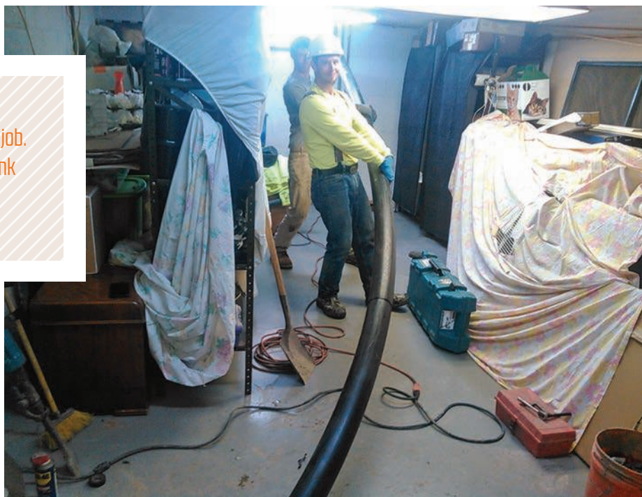
▲ A crew from R.I.C. Plumbing in Lockport, New York, holds the new HDPE pipe being inserted into an existing pipe lateral where crushed stone had collapsed in. Crews used a vacuum excavator with its hose attached to the end of the HDPE pipe in order to vacuum out the crushed stone and push the HDPE pipe through.
