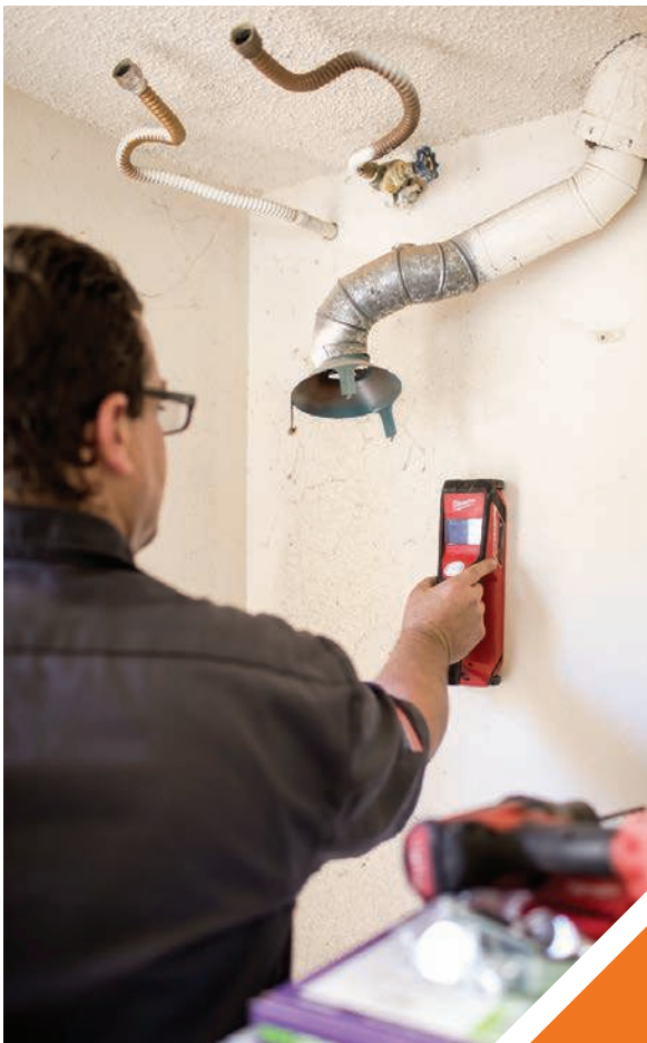
▲ Colgan searches for the wall studs while preparing to install a new water heater for a residential client after the old heater's tank failed. Colgan updated all aspects of the new water heater and its installation to the new plumbing codes including a drain pan, straps and fittings.
