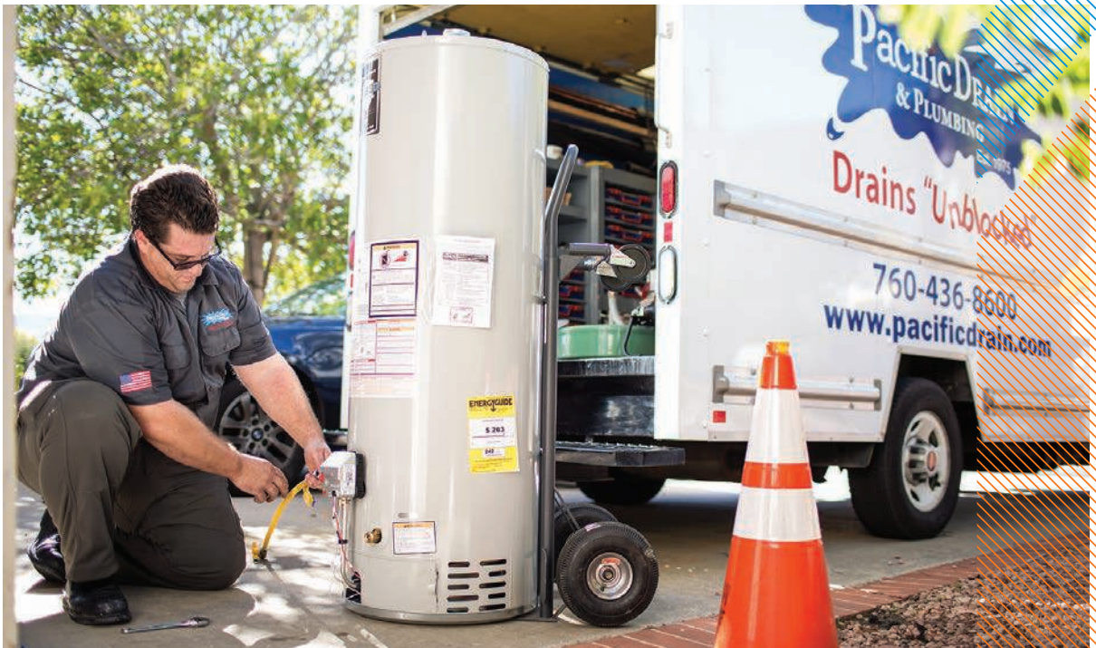
▲ Ryan Colgan, service technician, attaches the gas line on a new Defender water heater (Bradford White Water Heaters) in a driveway prior to installation at a client's home in San Diego.
