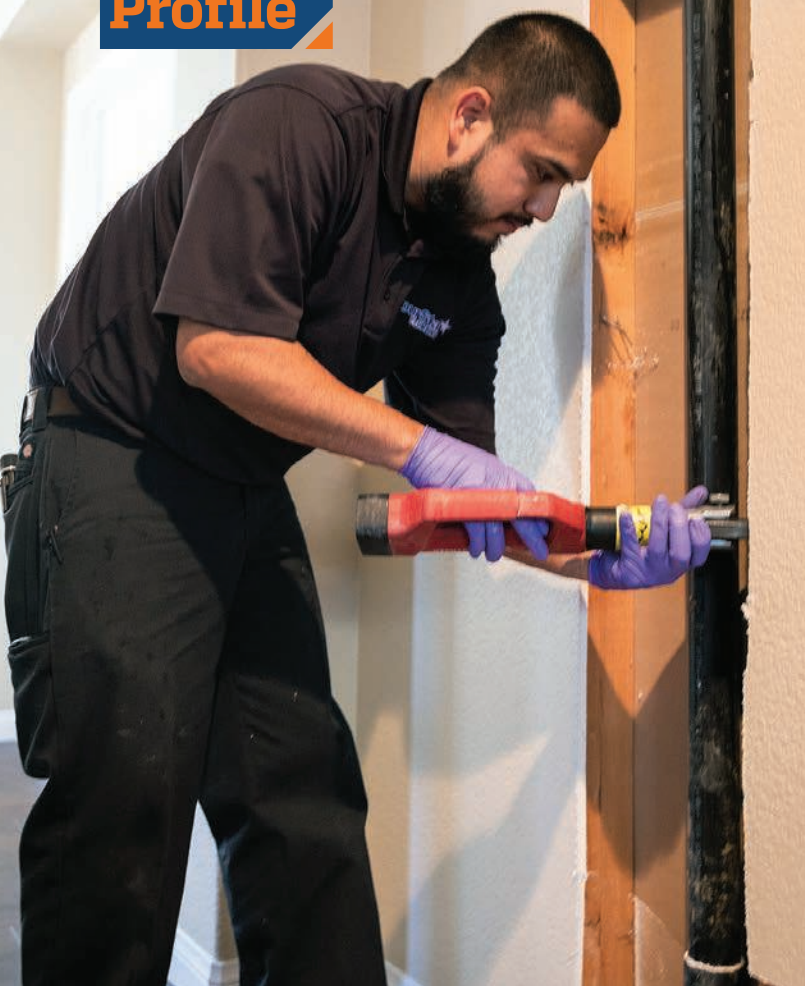
▲ Technician Angel Salgado uses a ROTHENBERGER USA crimping tool to begin his repair on a copper pipe, using 1/2-inch copper couplers that are crimped rather than needing to be soldered.
