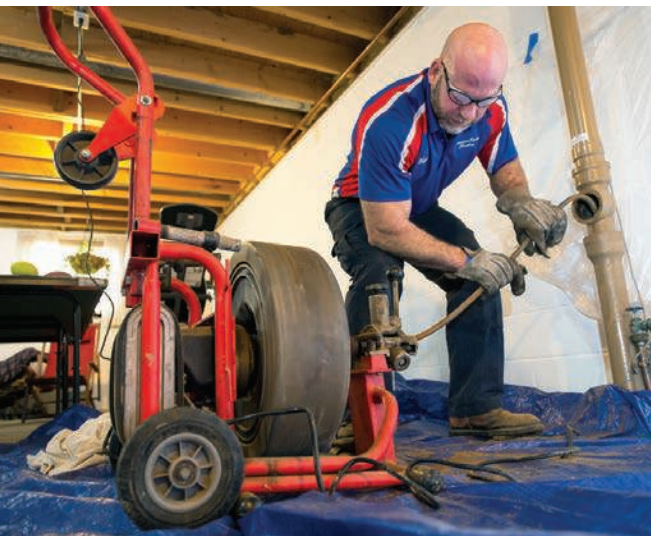
▲ Conn uses a RIDGID drum machine to remove roots during a drain cleaning job.
