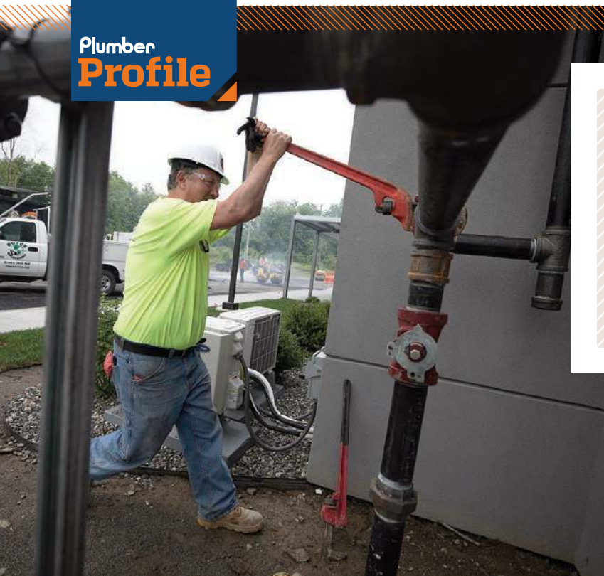
▲ Plumber Jim Cusanello works with a gas pipe in Middletown, New York.
