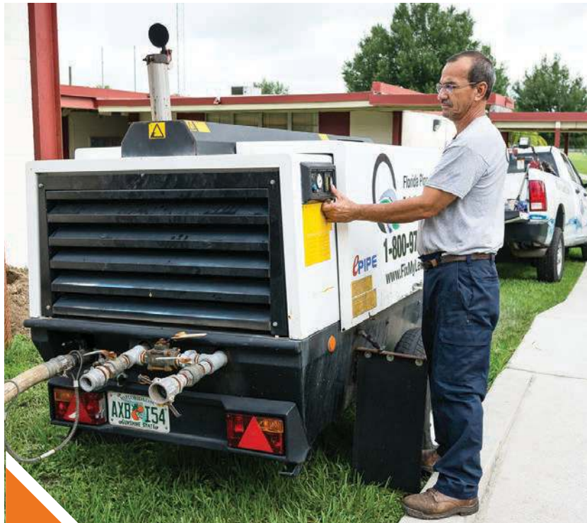
▲ Technician Javier Martinez works with an Atlas Copco Compressor during an ePIPE project.
