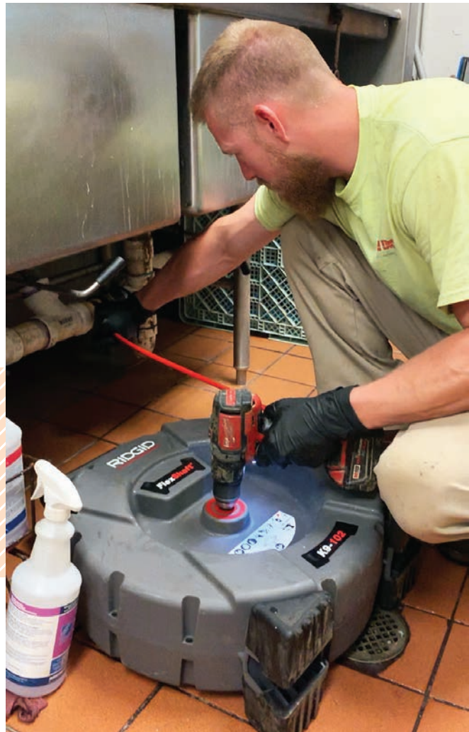
▲ Duane Goodpaster, owner of All Drains Drain Cleaning and Plumbing Repair in Ohio uses a RIDGID FlexShaft drain machine at a restaurant job. Goodpaster now owns four FlexShaft machines, two K9-102s and two K9-204s. (Photo courtesy All Drains Drain Cleaning and Plumbing Repair)
