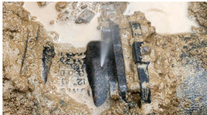
▲ A leak in a high-pressure waterline is exposed after detection and excavation.
