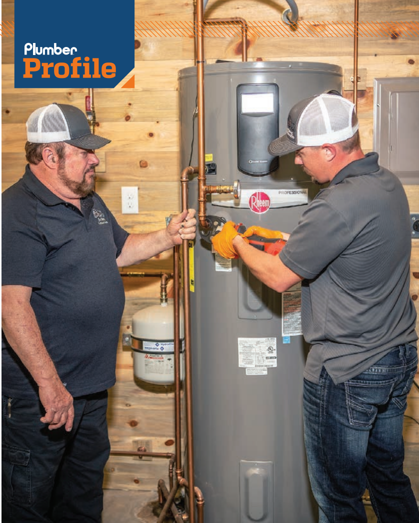
◆ Carl Keller, left, and Jeff Keller install a Rheem water heater at a residence in Jefferson, Texas.
