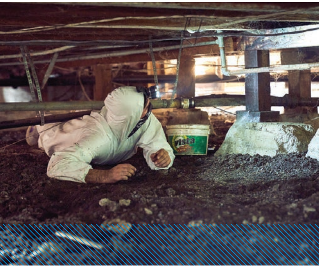
▲ Plumbing assistant Jeremiah Anthony crawls under a residence as he prepares to connect a new tankless water heater to existing water and gas lines.
