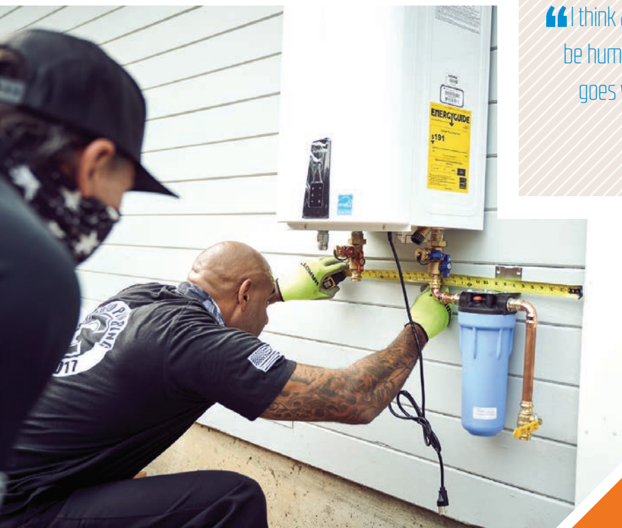
▲ Plumber Isaac Byrd measures to find the length of pipe he needs for installation of a new tankless water heater, plumbing assistant Jeremiah Anthony looks on.
