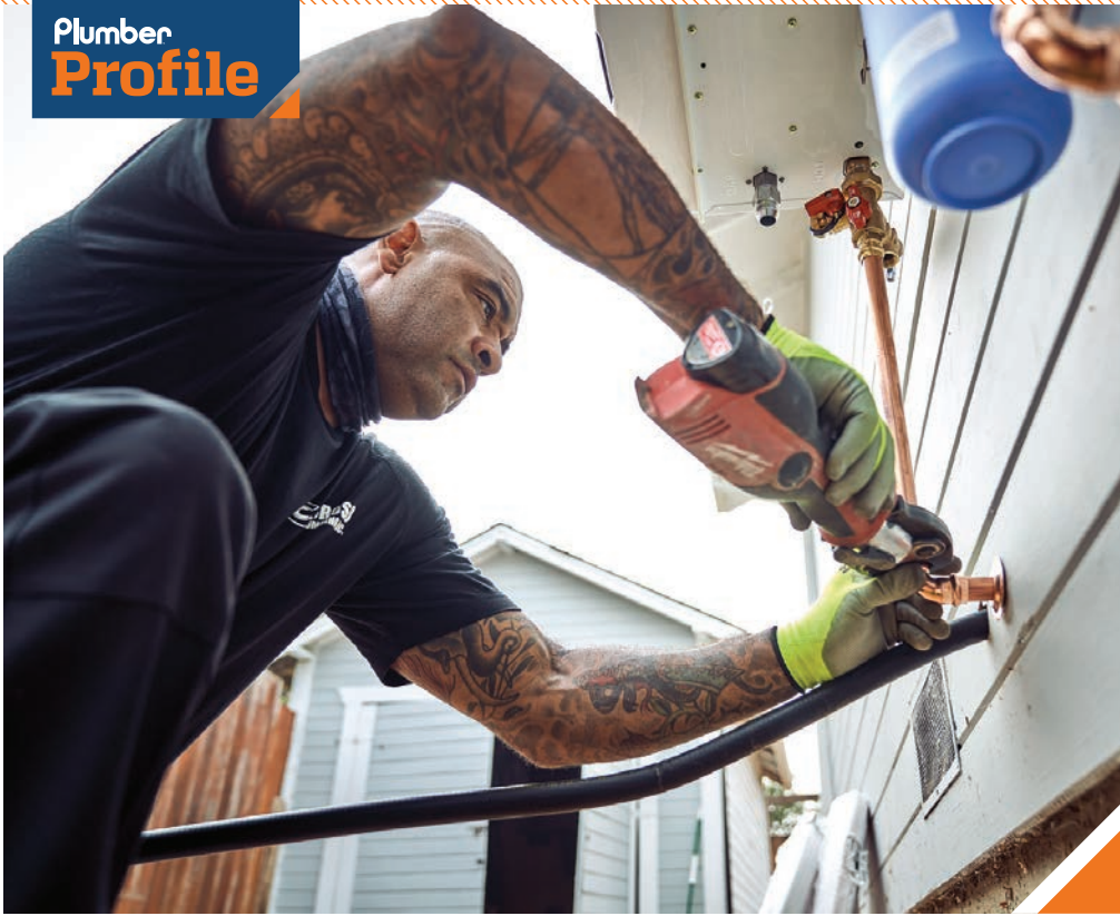
◀ Plumber Isaac Byrd presses together copper pipe pieces during a water heater installation job.
