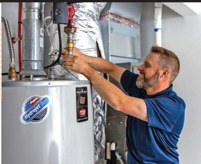
▲ Josh Knowlton works on a water heater installation at a customer's house who called the company after hearing their radio commercials.
