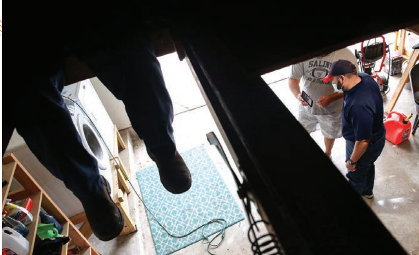
▲ Master plumber and service manager Jonathan LeBron, right, talks with a customer as Daisy Herrera, a journeyman technician, waits in the attic to complete a water heater repair at a home in Katy, Texas.
