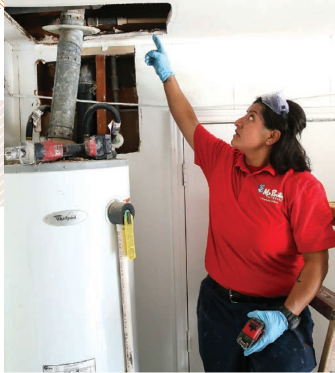
▲ Journeyman technician Daisy Herrera walks a customer through how they will repair a leak.
