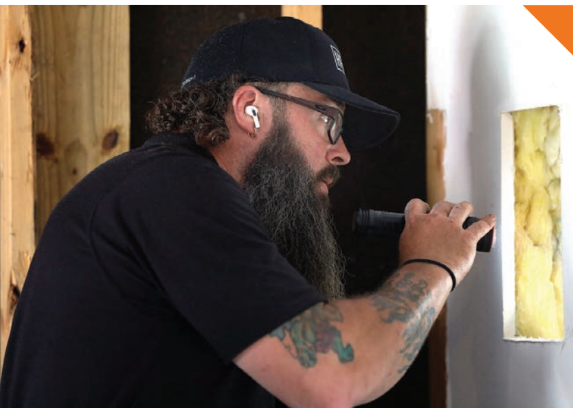
◀ David Hesson checks out the job after cutting out a piece of drywall where he will be installing a new shower valve in a home.
