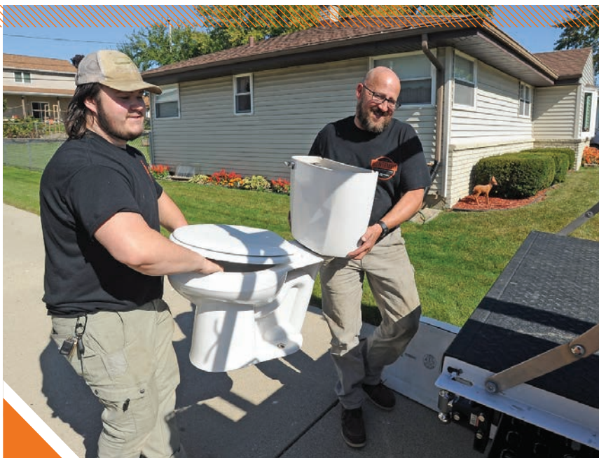
▲ Chris Bontempo, right, and Zach Bajewski load up an old toilet from a residential property. Bontempo was hired to replace the old toilet with a new Kohler toilet.
