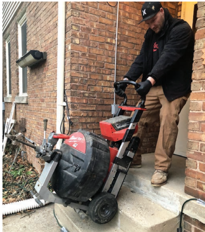
▲ Drains R Us of Southeastern Wisconsin technician Kenny Szczesny guides the Milwaukee Tool MX Fuel drum machine with POWERREDZ stair-climbing, lift-assist technology into a customer's home. (Photo by Ken Wysocky)
