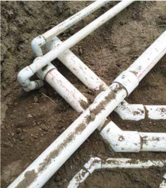
▲ In this photo of a koi pond under construction, the first contractor on the job laid the pipe with too many angles, which created friction and less movement of the water to filter the pond. A repipe was required. (Photo by James Careless)
