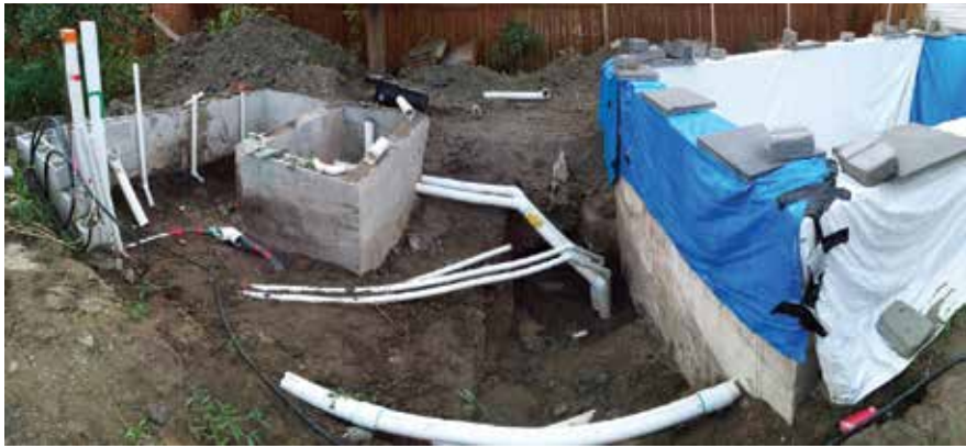
▲ The best koi pond designers use a wide diameter pipe, like 4-inch or larger, with no angle fittings. If corners need to be made, they should be 90 degree sweeps or flex pipe.
