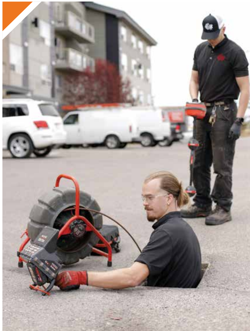
▶ Journeyman plumber Isaiah Baker uses a RIDGID CS6X SeeSnake and RIDGID MINI TruSense while apprentice Peter Baker, back, uses a RIDGID Navitrack as they perform a sewer inspection.
