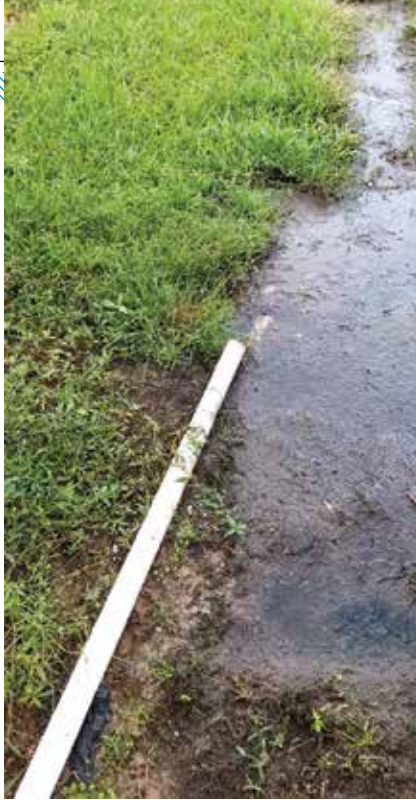
▲ A simple fix for many of those homeowners in Lowndes County was to install "straight-pipe" systems — a pipe connected to the home's building drain and piped straight to ground surface.
