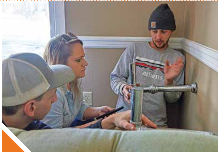
▲ Lindsay Goodson, center, along with fellow plumbers Bobby Lane, left, and Lincoln Vincent analyze the pipe connection at an installation project.
