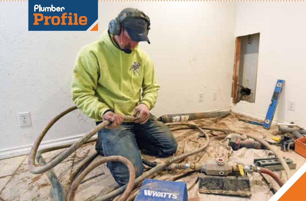
◀ J.D. Christensen disconnects an air hose from the Vermeer pneumatic hole hammer that the team is using during an installation project.
