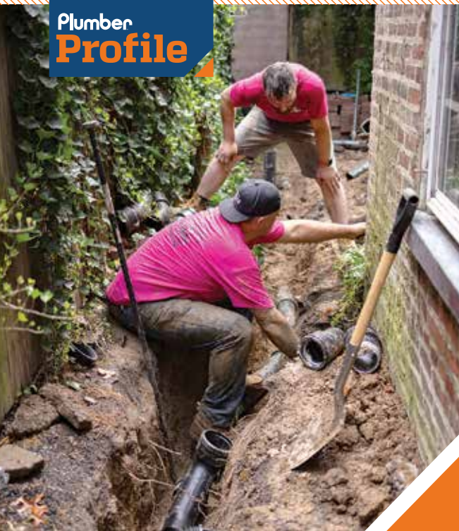
▲ Anthony Alfonse, a plumber with John Snyder Plumbing & Heating, looks on as John Snyder works on the installation of new pipes. The company has a total of four employees.
