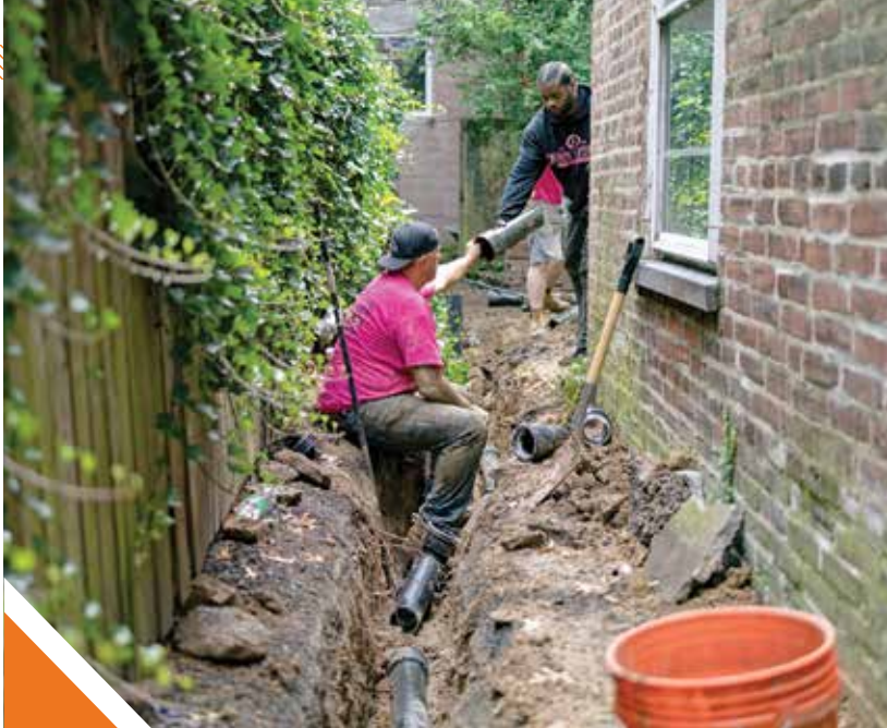
▲ Plumber Khalil Reed hands John Snyder a section of cast iron pipe for installation.
