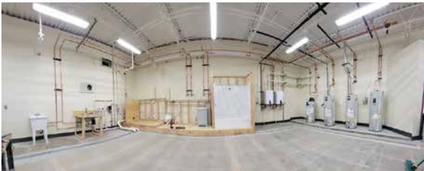
▲ Photo of the new Navajo Technical University plumbing lab located in Crownpoint, New Mexico.
