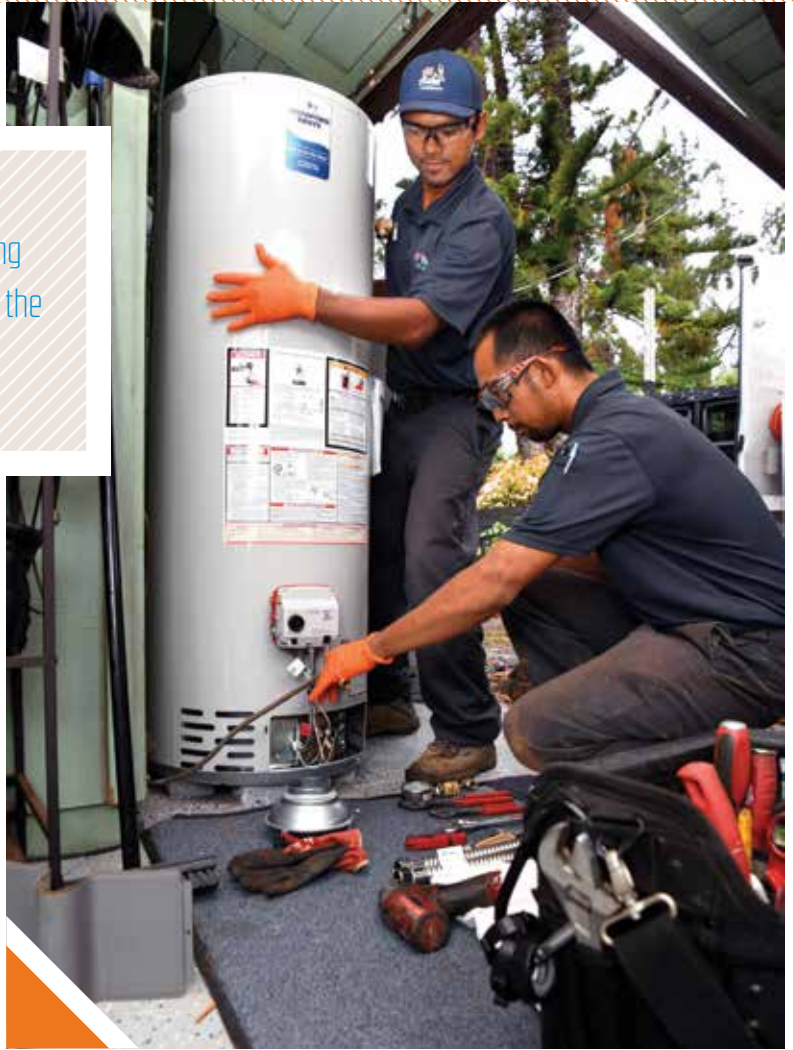
▲ Kenny Agdinaooy, kneeling, and apprentice Ben Garcia install a new propane water heater (Bradford White).
