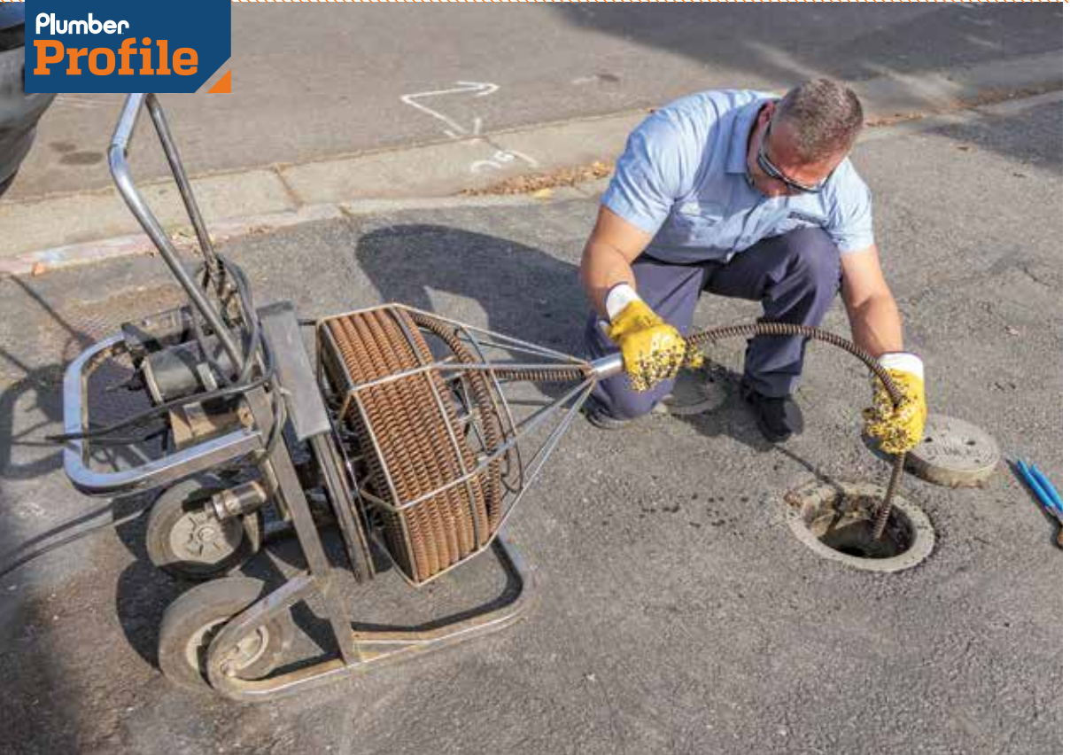
▲ E.J. Jimenez works with a Quadra Plex 2000 cable drain machine on a residential plumbing job near Santa Clara, California. (Photography by David J. Elkins)
