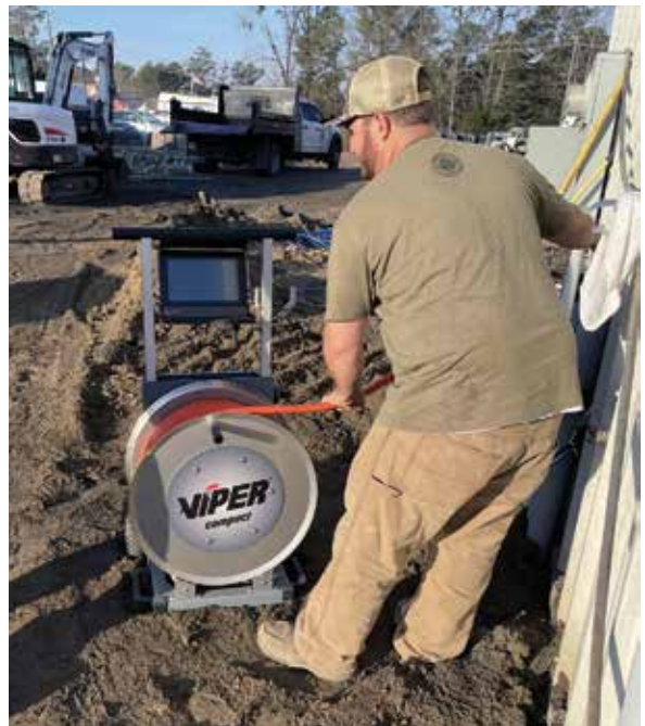
▲ Mason Powell, a technician for Stokes Plumbing & Trenchless, uses a Viper combination camera and jetter to inspect and clean a 36-inch-diameter stormwater sewer at a business in Georgia. (Photo courtesy of Stokes Plumbing & Trenchless)
