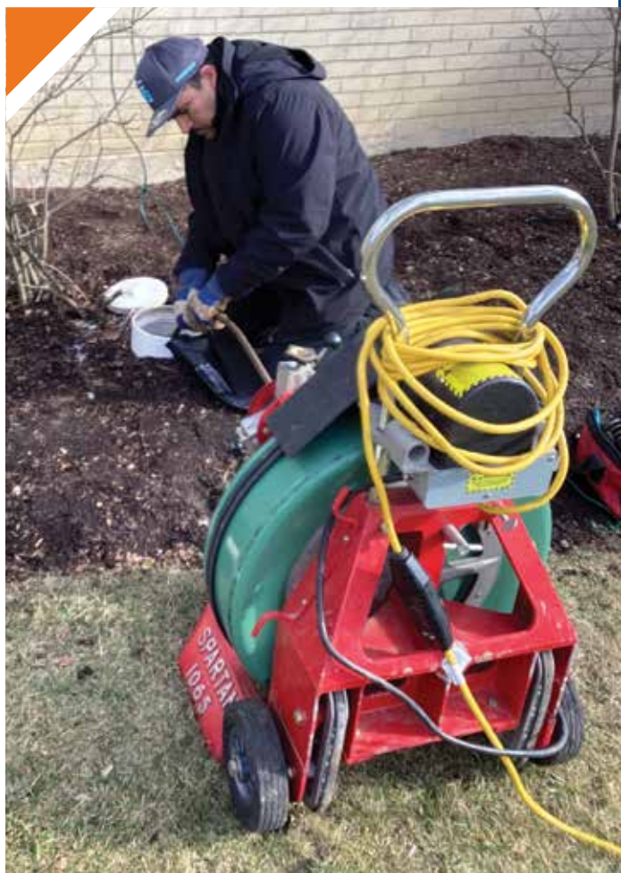
▲ Plumber Javier Gutierrez uses a Spartan Tool 1065 drain cleaning machine on an outside drain as a residential property. The company's plumbers have Spartan Tool and RIDGID drain cleaning tools on their work vans to be ready for any job.
